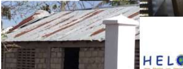
Roof of our primary school/church, mostly in tact with the exception of the far end.
